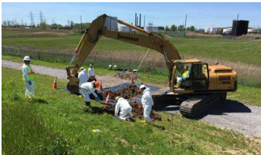
Excavating a test pit in the Seaway FUSRAP site. U.S. ARMY CORPS OF ENGINEERS
