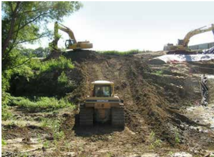
Cleanup at the St. Louis Airport Site. U.S. ARMY CORPS OF ENGINEERS
