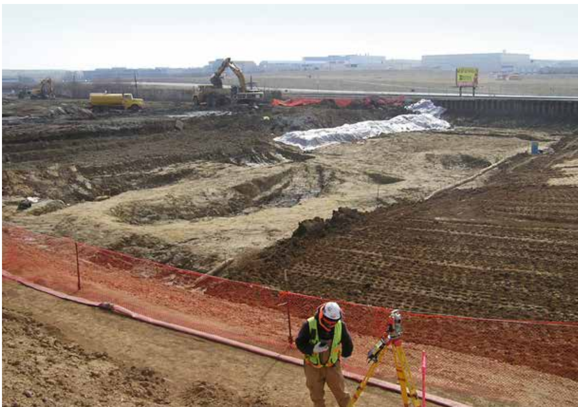
Cleanup at the St. Louis Airport Site. U.S. ARMY CORPS OF ENGINEERS
